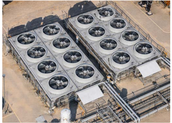
Overhead view of fin fans systems at the Vistra Corp energy facility.
